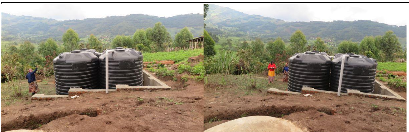
4 Tanks of 10.000 that are collecting water from all the roofs
